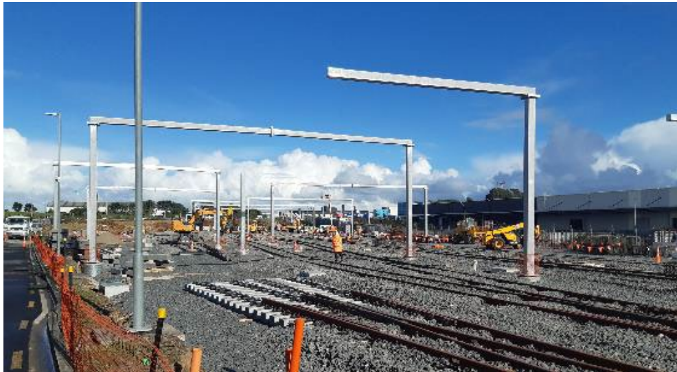
Wiri Train Stabling Yard construction underway and will be ready to receive first of the new trains in July 2024
