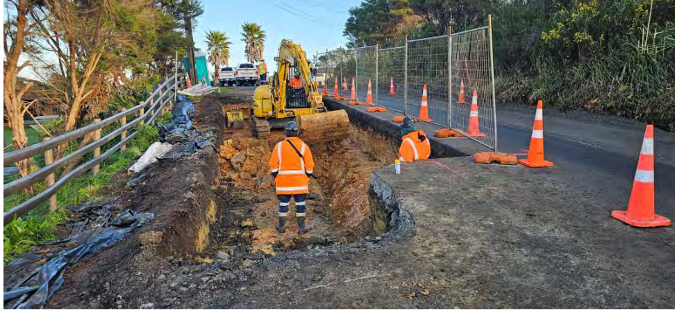
Damaged material being removed from under the pavement on Wairere Road, at Roster Ridge.
