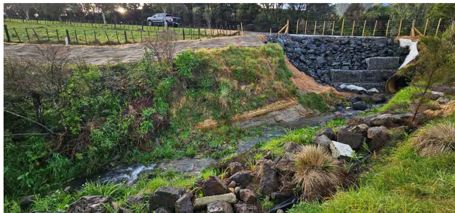
Slip repair on Gum Road Henderson Valley
