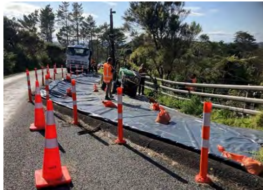
Wairere Road slip site 349 Wairere Road
