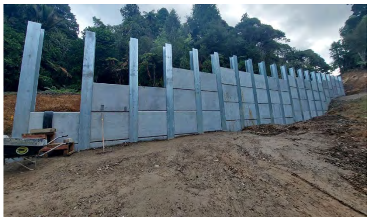
Retaining wall construction on the site on Scenic Drive, just past Arataki
