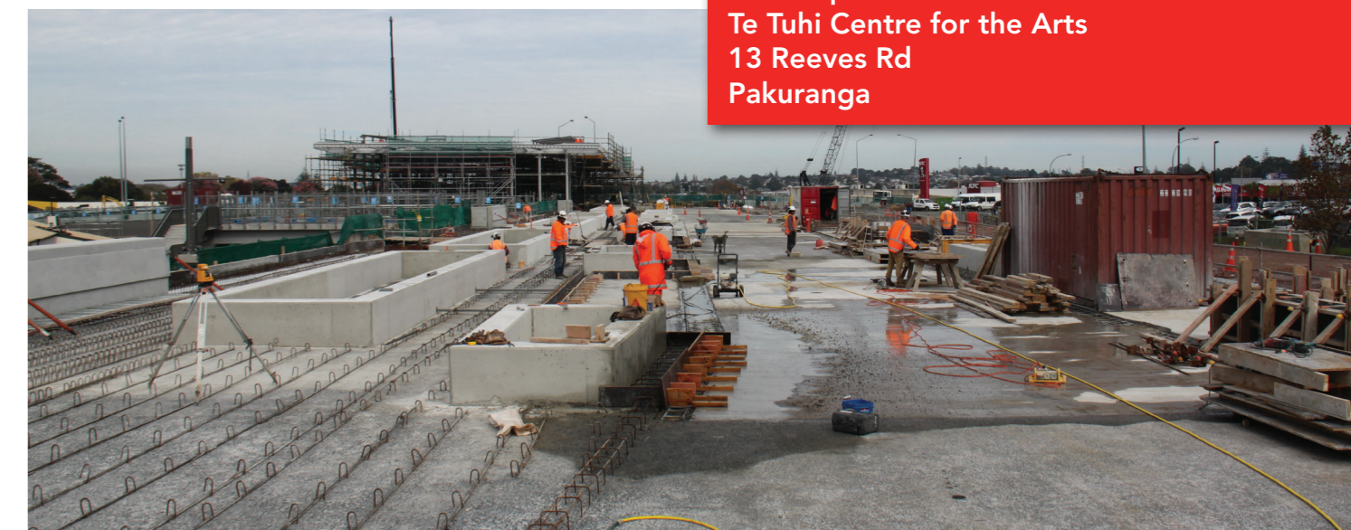
Above: Construction of new AMETI local road on top of tunnel to be used as an interchange for easy transfers between trains and buses with new Panmure Station in background.
