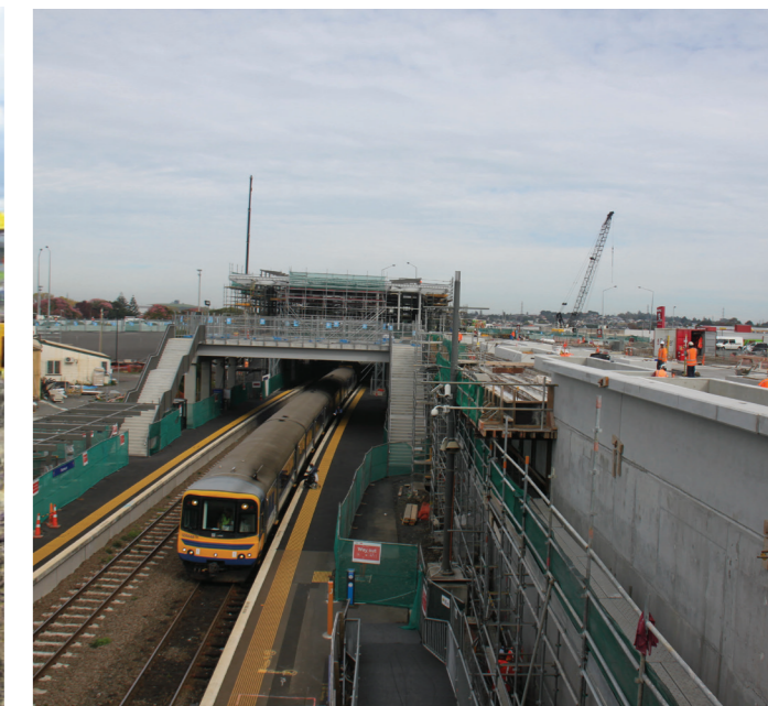
Photo top right: Work continues on the laying of new communications cabling at Panmure Station.
