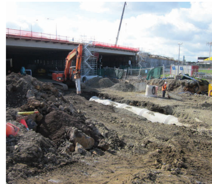
Photo top left: Excavation has started for the AMETI link road south of Ellerslie-Panmure Highway, with a large new stormwater culvert being placed under the length of the road.
