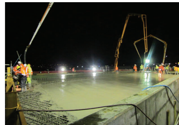
Photo bottom left: Concrete deck poured for the new Ellerslie Panmure Highway bridge.
