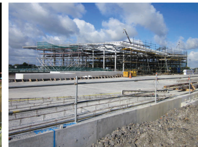
Photo bottom right: The new station building wrapped in temporary scaffolding whilst work takes place on the roof. The new local road and planter boxes are visible in the foreground.
