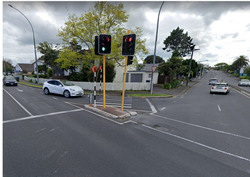
Existing traffic island deficiency at St Lukes Road/Morningside Drive intersection
