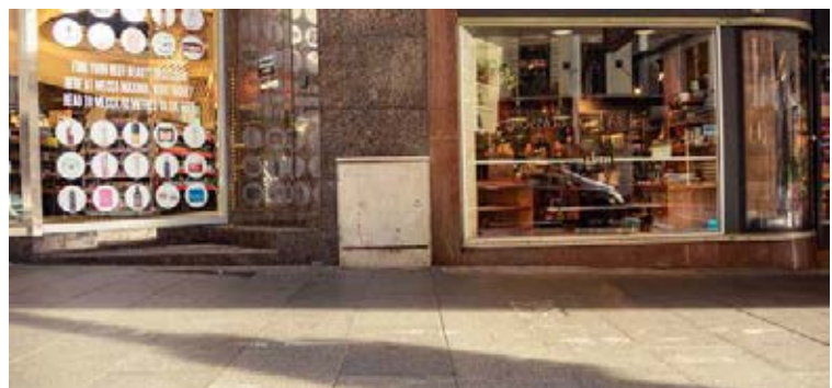
Figure 7 Good practice Narrow cabinet flush to building line, and clear of door and corner of building, within frontage zone
