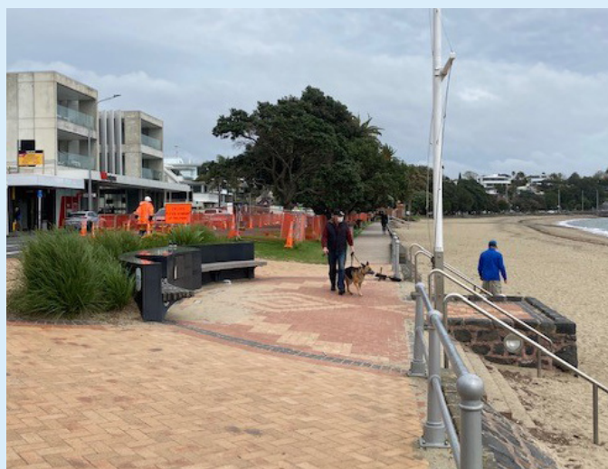
Pedestrians out enjoying the greater freedom of Level 3, while work starts back up on St Heliers safety improvements Stage 2
