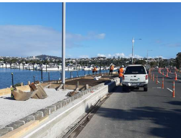
AT has raised the height of the Tāmaki Drive seawall to improve resilience to sea level rises
