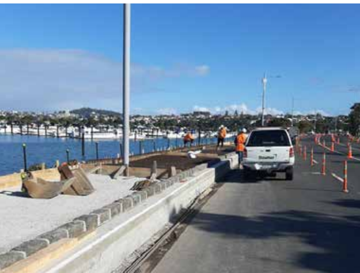
AT has raised the height of the Tamaki Drive seawall to improve resilience to sea level rises
