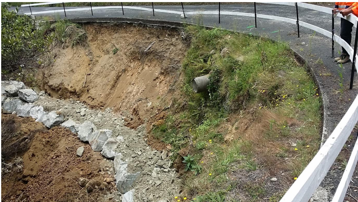
Slip damage in Aotea.
