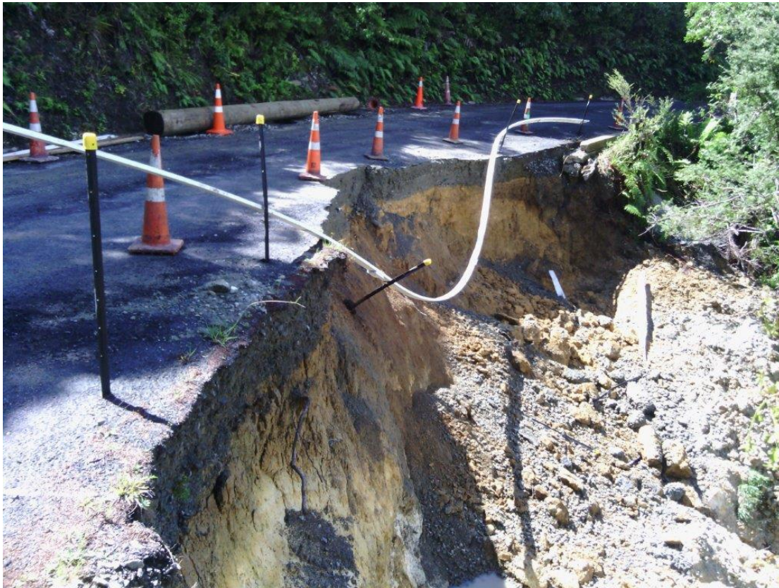
Windy Canyon – Additional damage from Cyclone Pam.
